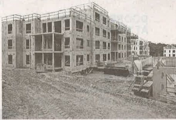
Work continues for the St. Regis Residences, which have already attracted interest among buyers. PHOTOS BY MARK VERGARI/THE JOURNAL/NEWS
